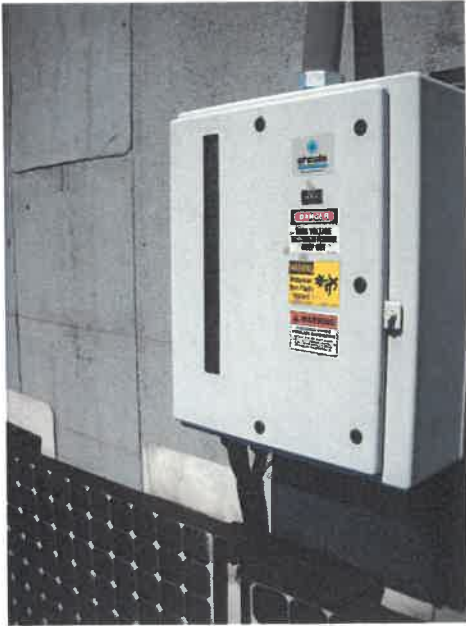
Figure 3-27 Rooftop DC Combiner Box
