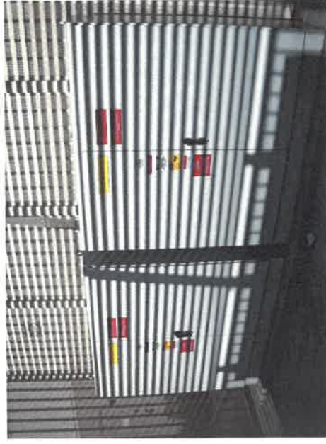
Figure 3-30 DC Fuse Box at San Bernardino
