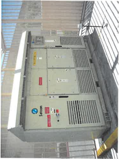
Figure 3-31 DC to AC Inverter at San Bernardino
