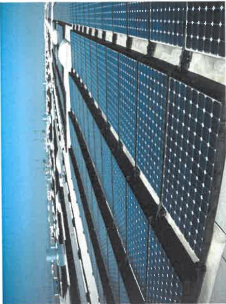
Figure 2-9 Solar Panels on Rooftop Facility
