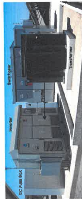
Figure 3-17 Measurement Profile Path Between Transformer and Inverter at Porterville
