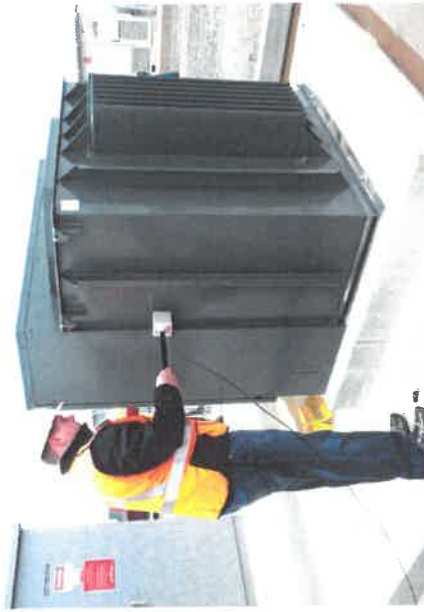
Figure 4-12 Measurement of Electric and Magnetic Fields near the Surface of Transformer 02 at the Porterville Facility - A fiber optic cable connects the sensor to a laptop computer that runs the analysis software.
