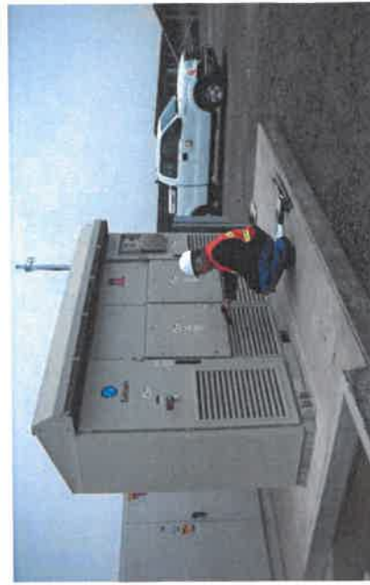
Figure 3-15 AC Magnetic Field Measurements at Front Base of Inverter at Porterville
