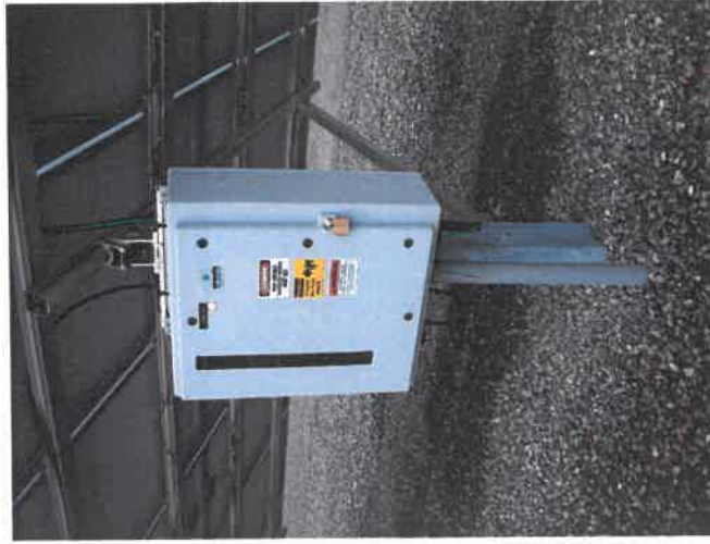
Figure 3-9 Photograph of a Combiner Box at Porterville
