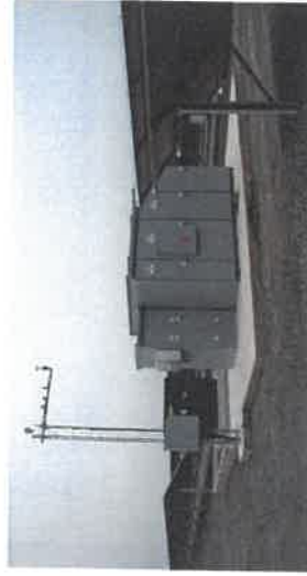
Figure 3-19 Switchgear at Porterville Solar Farm
