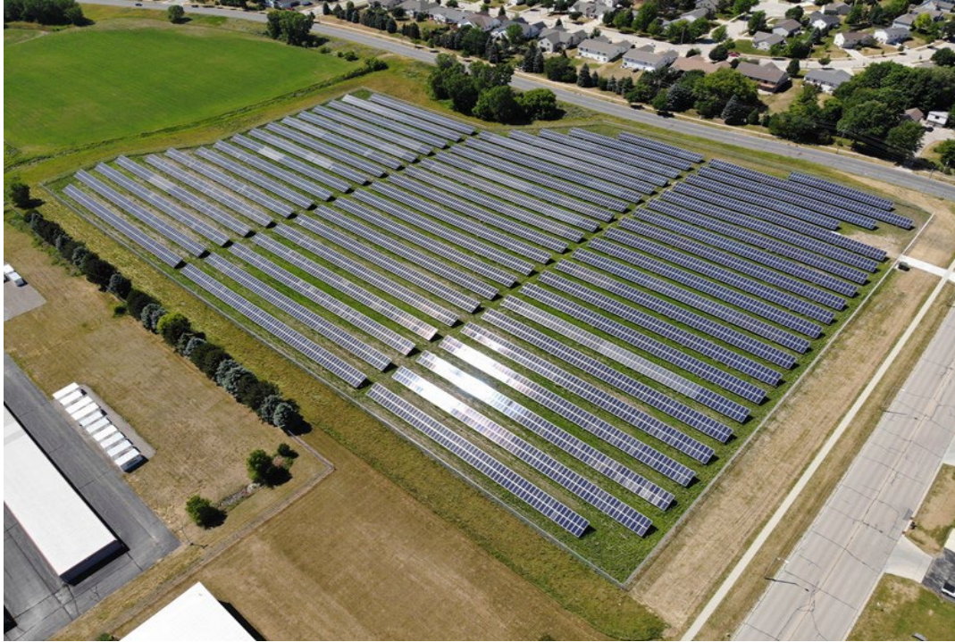
Figure 2 - Example of a solar array with an establishing pollinator habitat
