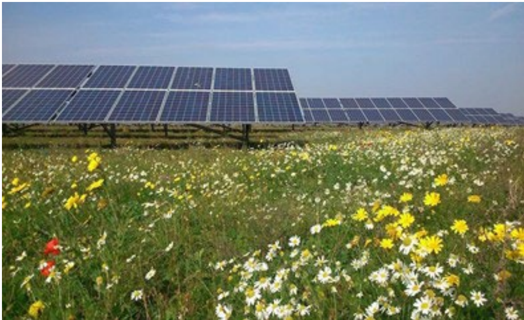
Figure 3 – Photo of a fixed mounted solar project with established native vegetation
